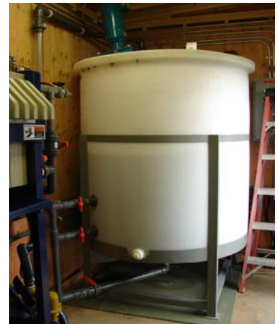
Figure 2 – Reactor Tank & Mixer
